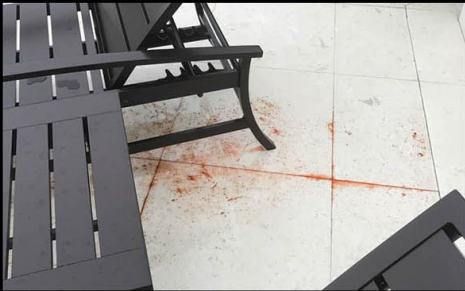
Rust comes from steel screws or frames.
