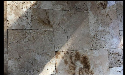
Sand set installation using sand contains iron deposits causes rust stain.
